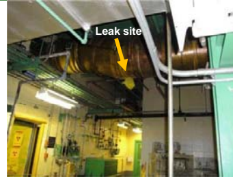
Area where contaminated duct was remediated
