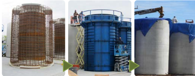
Concrete casks will surround steel inner-liner. Concrete cask fabrication will take place at the WVDP.
