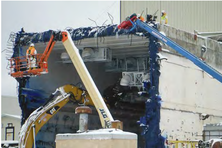
Crews lower a cooler to the floor as part of Vitrification Facility demolition activities.
