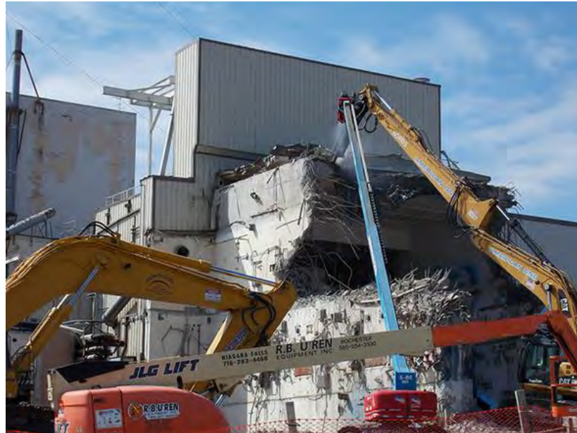
Workers tear down a portion of the Vitrification Facility containing a process cell.
