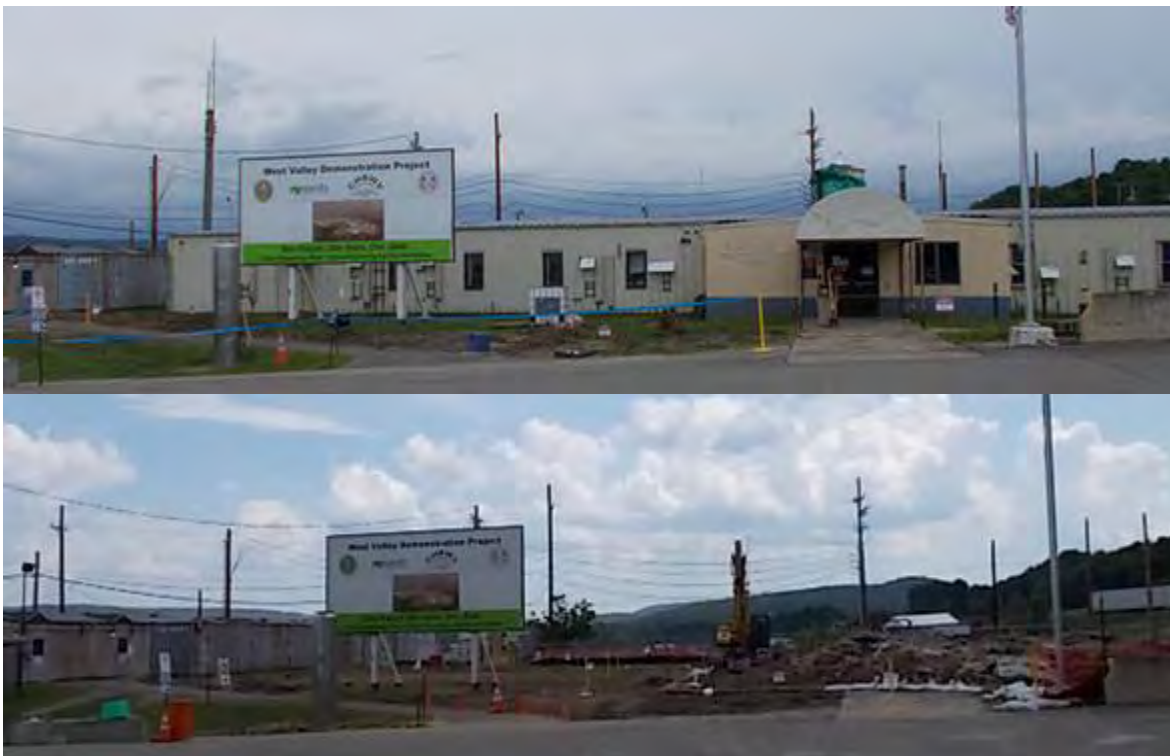
Before and after: The West Valley Demonstration Project site's footprint is dramatically changed following demolition of the former administration building.
