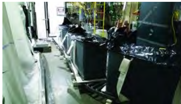
Three 900-pound lift bags filled with ACM sit on the employee-designed conveyor system used to improve safety and increase efficiency.
