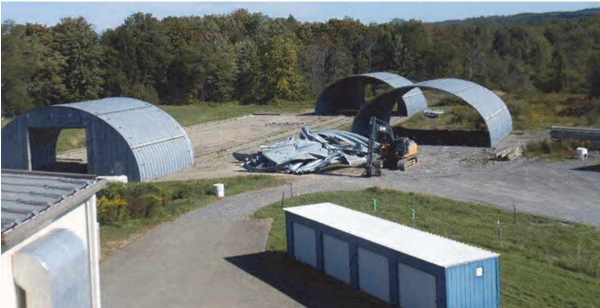
Crews tear down sections of a former waste storage building. Debris from the demolition was loaded into waste containers and shipped off-site for disposal.
