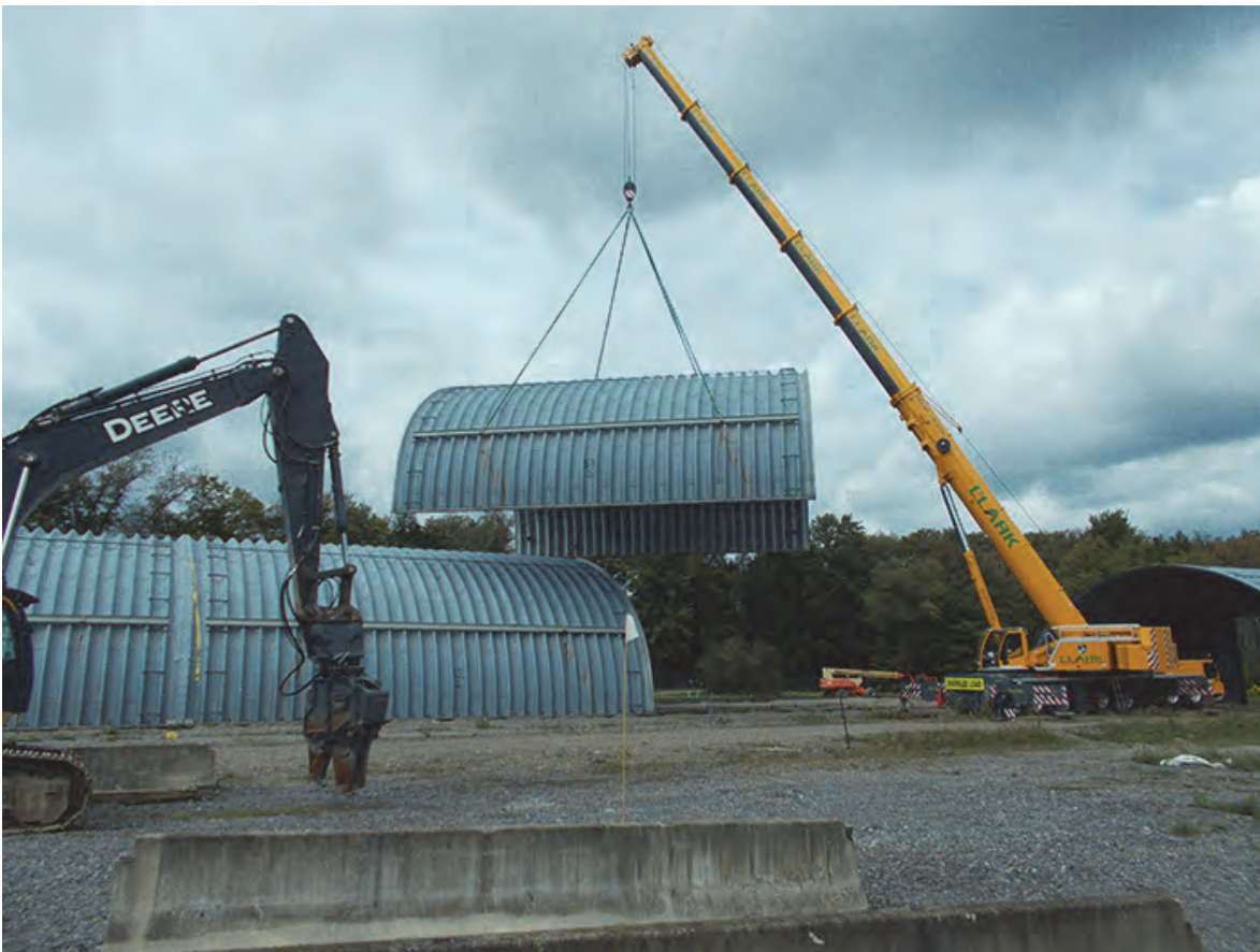
A large crane is used to relocate sections of a former waste storage structure for safe demolition at EM's West Valley Demonstration Project Site.
