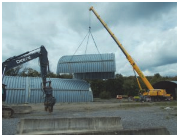
A large crane is used to relocate sections of the CPC-WSA to an area where they can be safely demolished.
