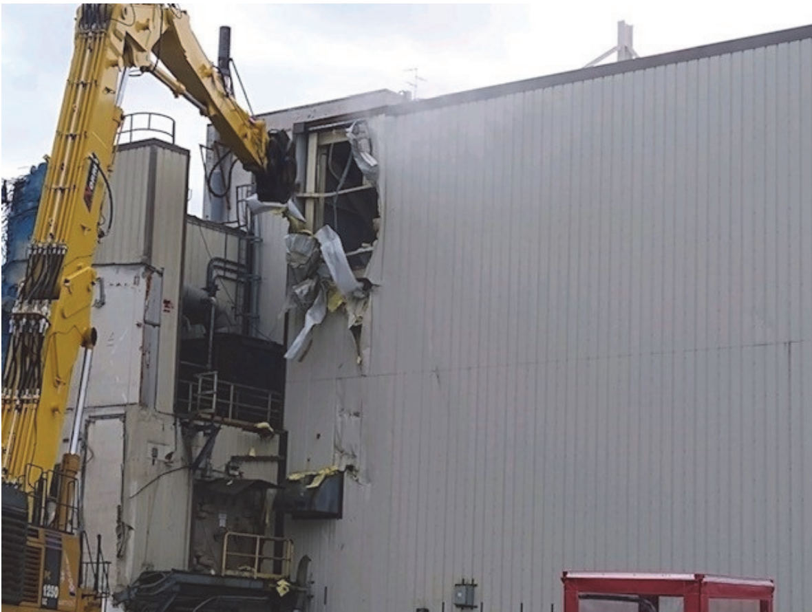
A view of the start of demolition of the Load-In Facility, the last of seven buildings that supported operations at the former Main Plant Process Building at the West Valley Demonstration Project .
