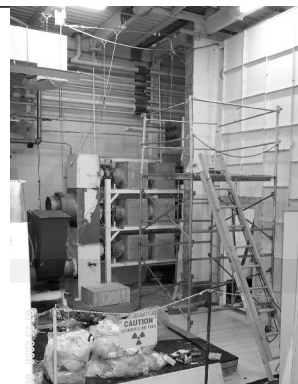
The XCR will be cleaned out to provide access to PPC below
