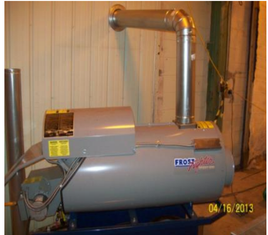
New Utility Room Natural Gas Heater
