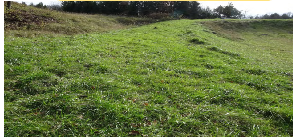
Lake 2 Overflow Flume Needs Reshaped to Slope in Opposite Direction
