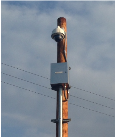
Security Cameras Installed
