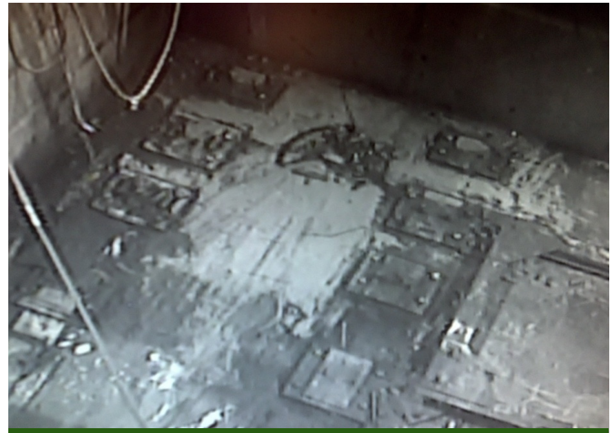
Vit Cell Equipment Pit East Side After Vacuuming
