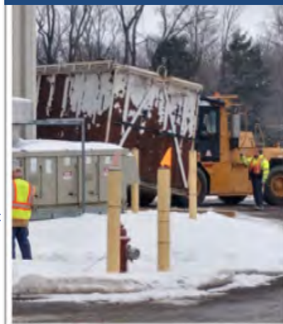
A large box containing the Dissolver is transferred into the Remote-Handled Waste Facility
