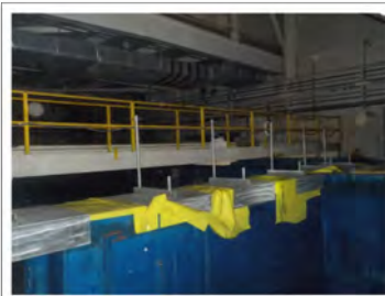
Fuel Receiving & Storage Area
