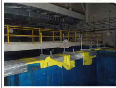
Fuel Receiving and Storage Facility
