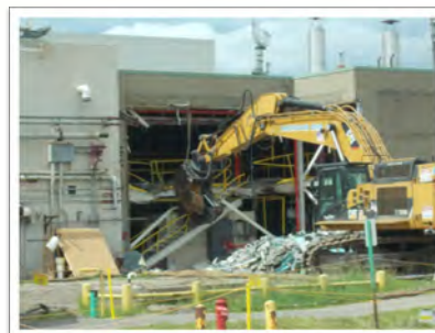
An excavator with a shear attachment is used to remove the stairs in the Utility Room Extension building during demolition
