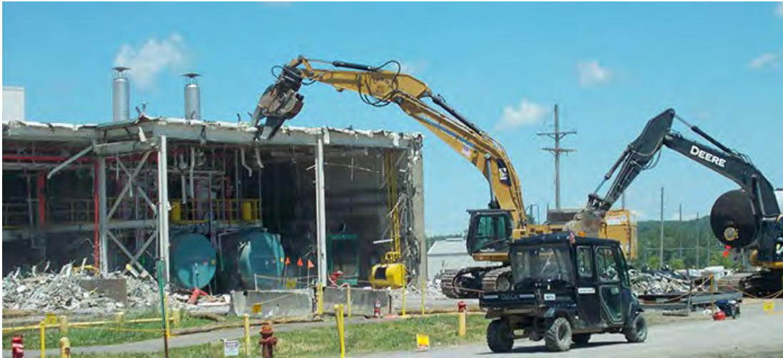
A crew demolishes two boilers at the former utility room extension building. Workers then size-reduced and packaged them for off-site disposal.
