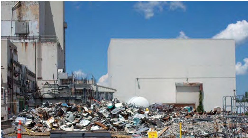
A view of debris following completion of demolition of the former utility room extension building.
