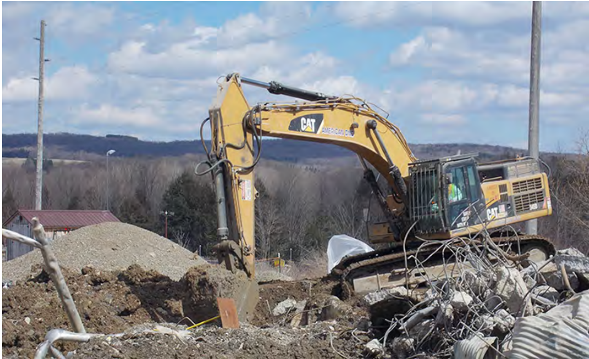
A large excavator digs near a sump that collected water from the drains of a facility formerly used to treat low-level waste.
