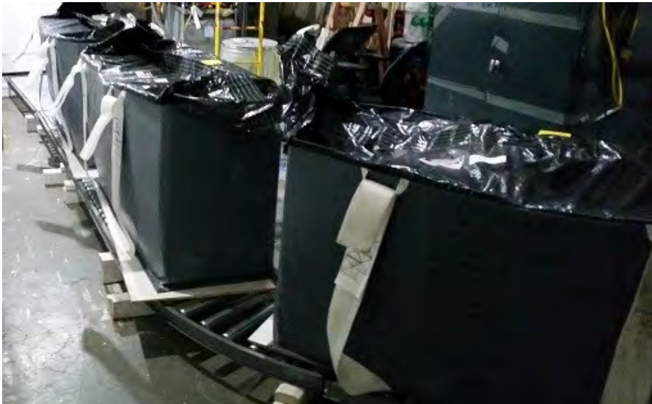
Three 900-pound lift bags filled with asbestos material sit on a conveyor system designed by workers at EM's West Valley Demonstration Project.
