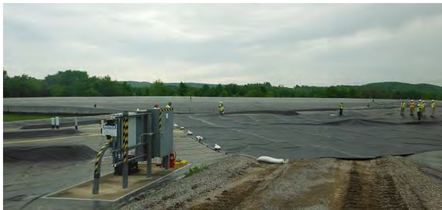
Workers position a temporary protective cover over the pretreatment system facility demolition area until a permanent one is installed later this year.
