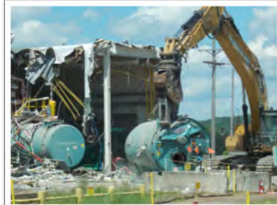
An excavator with a shear attachment is used to remove a boiler from the Utility Room Extension building during demolition
