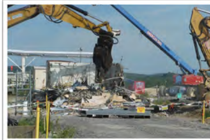
An excavator is used to demolish the Waste Tank Farm Equipment Shelter
