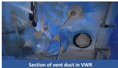
Section of vent duct in VWR
