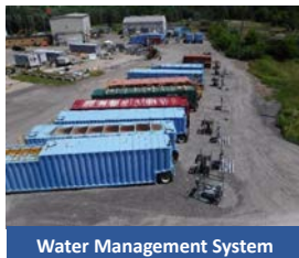
Water Management System
