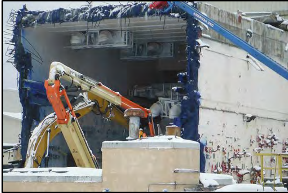
The first of four in-cell Vitrification Facility coolers is lowered to the floor as part of the removal process. This particular task was the highest remaining hazard associated with the Vitrification Facility project, and is critical to continuing with the demolition of the facility.
