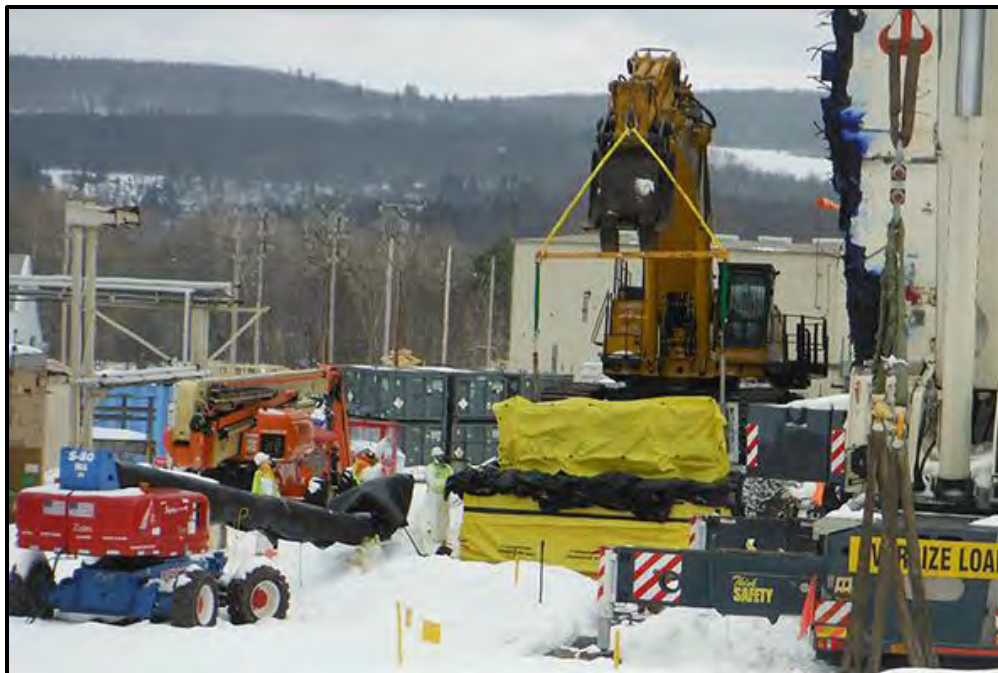
The second of four in-cell Vitrification Facility coolers, covered in yellow herculite, is lowered into a waste storage box. The waste box includes contamination controls and cribbing for safe transport and storage.
