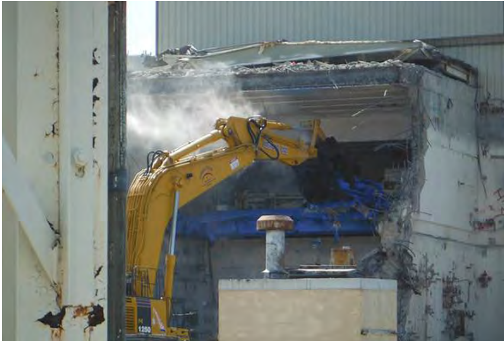
Crews demolish a portion of the West Valley Demonstration Project Vitrification Facility.
