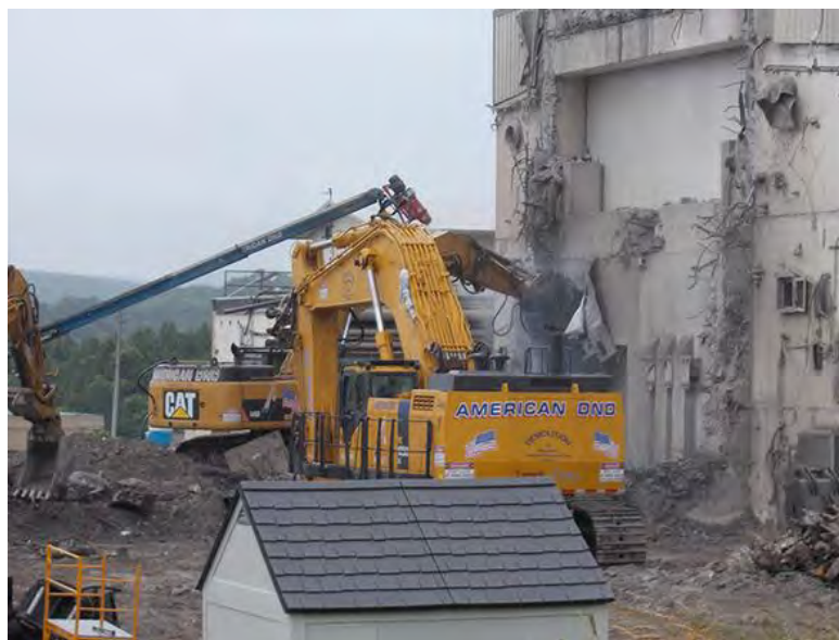
With the second phase of the Vitrification Facility demolition project complete, all that remains for removal is the south wall, shield doors, small cranes, and minor equipment.
