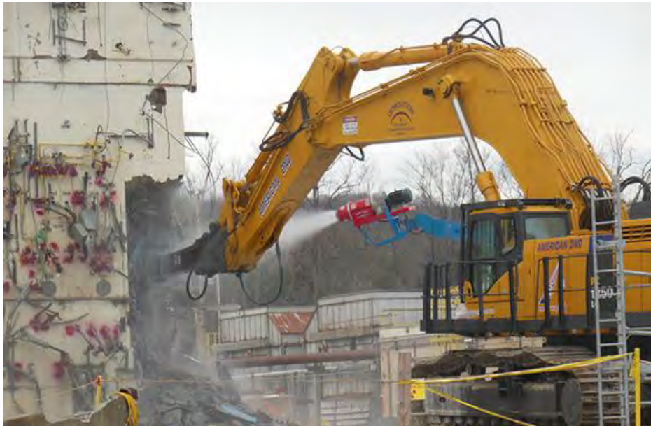
Crews take the “first bite” of the Vitrification Facility during the second phase of demolition.
