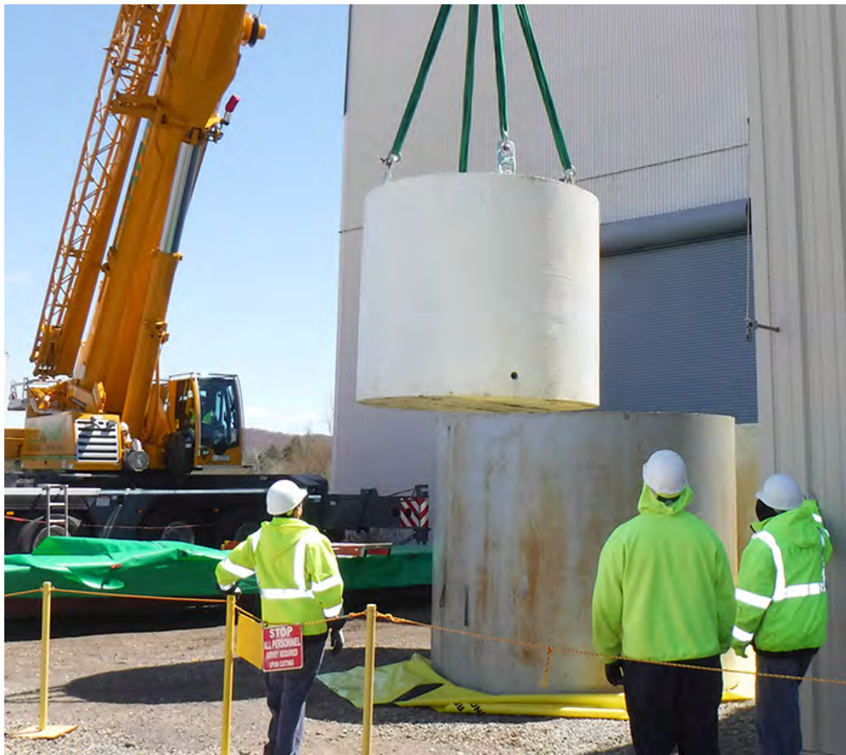
Using a 200-ton crane, workers return a waste container to its exterior steel shield at its new location at an outdoor storage area.
