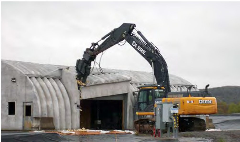
Demolition equipment takes the first bite out of a facility housing a liquid pretreatment system at EM's West Valley Demonstration Project.
