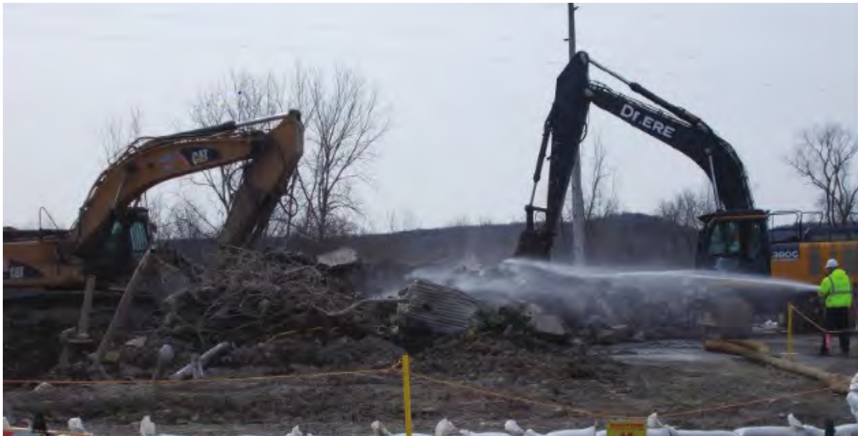
Two large excavators create work efficiencies as one demolishes the structure and the other size-reduces and loads debris.
