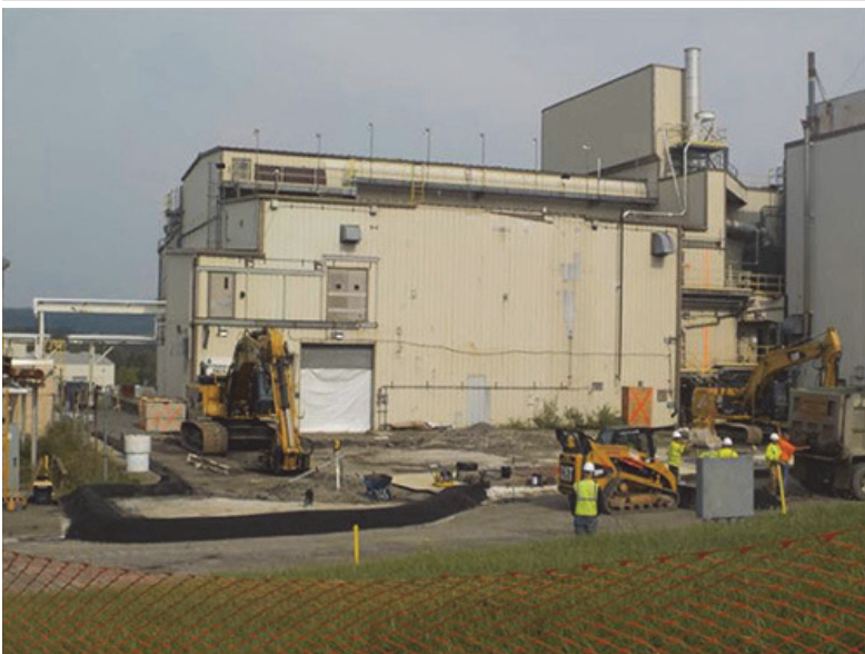
A view of the Vitrification Facility prior to demolition at the West Valley Demonstration Project. The facility was the largest and most complex demolition at WVDP to date. The WVDP team used lessons learned, best practices and a methodical approach to safely complete this major milestone.
