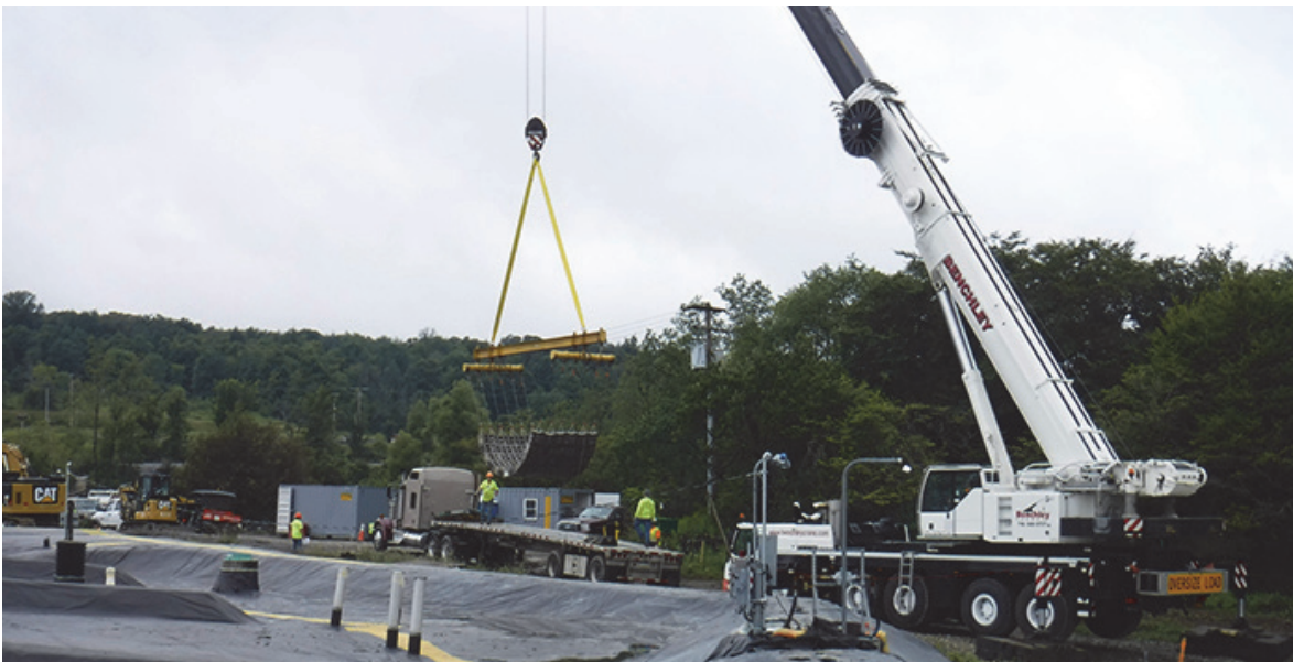
A crew moves a section of interlocking concrete blocks for placement at a closed disposal area at the West Valley Demonstration Project Site .
