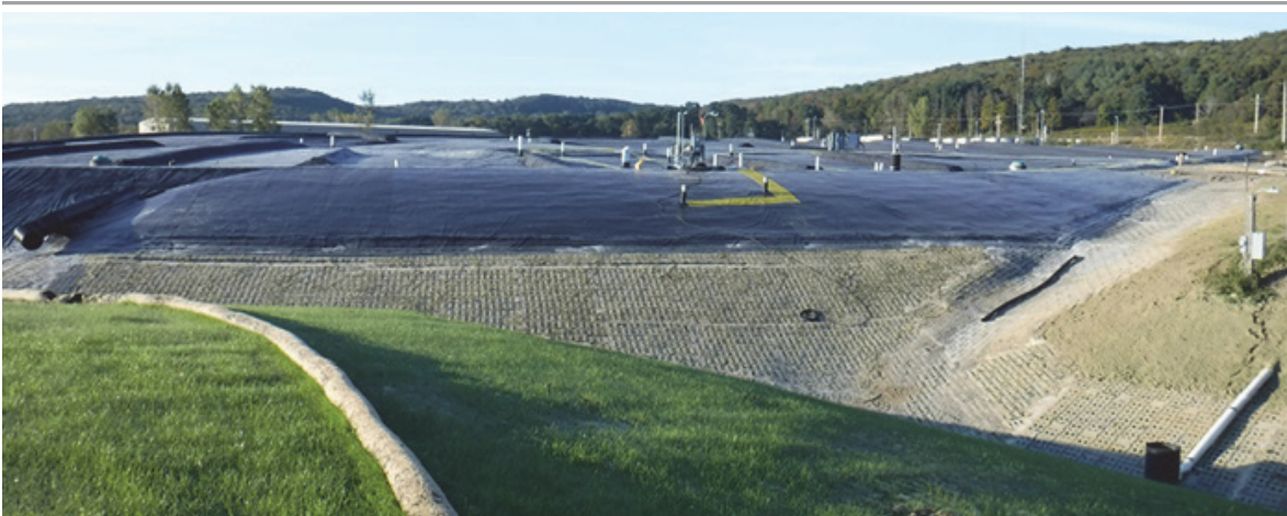
Workers installed interlocking concrete blocks to prevent erosion along a closed disposal area's north slope, pictured here, at the West Valley Demonstration Project Site .
