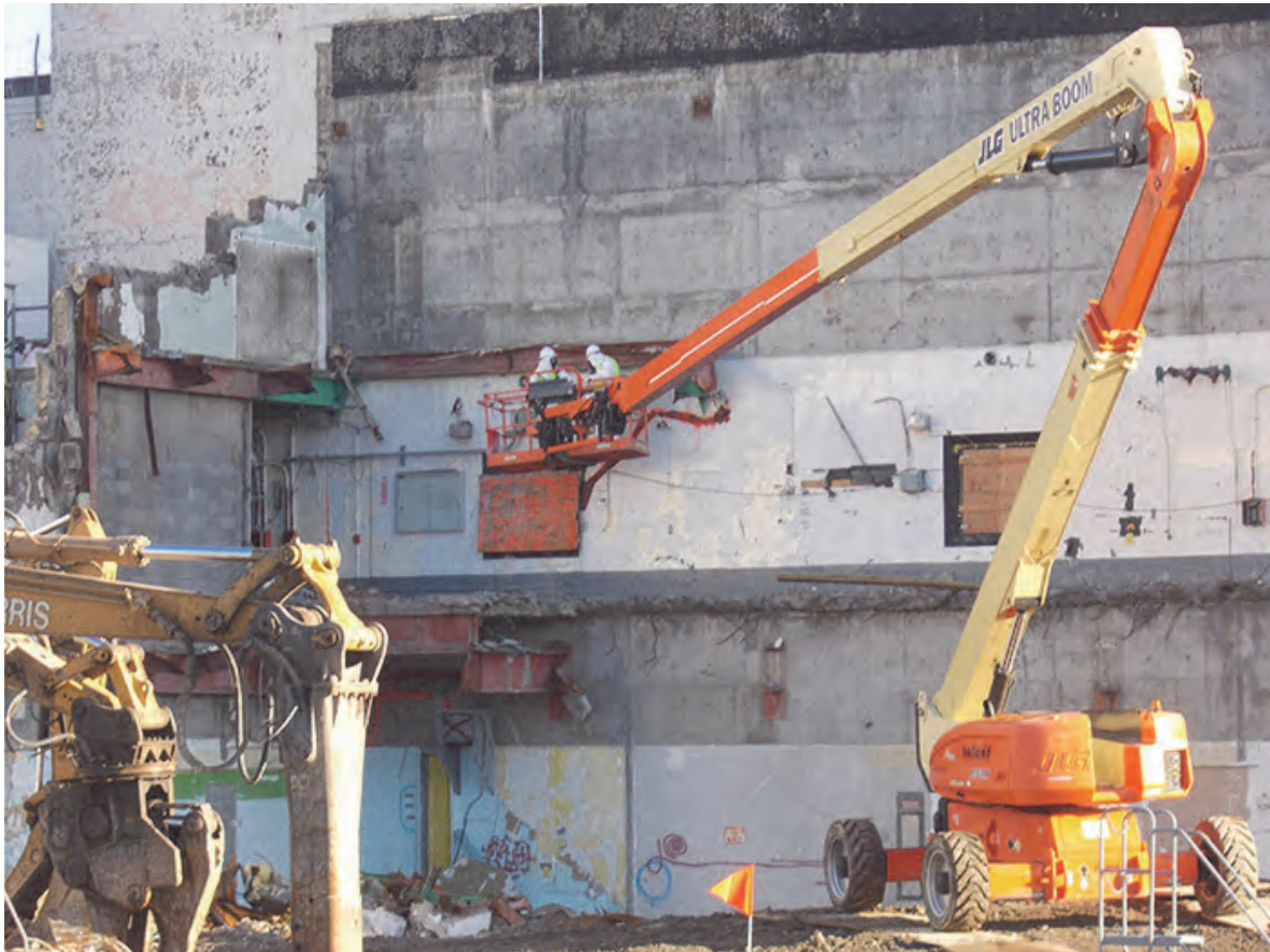
Radiation technicians from area small business InTomes survey of the exposed exterior wall of the Main Plant Process Building at EM's West Valley Demonstration Project Site after the demolition of the Main Plant Office Building.
