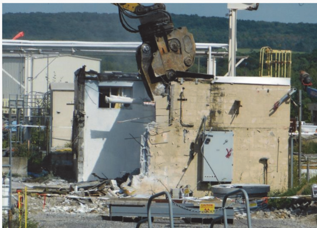
An excavator is used to start demolition of the waste tank farm equipment shelter in November 2019 after completing the removal of two condenser structures at the West Valley Demonstration Project.
