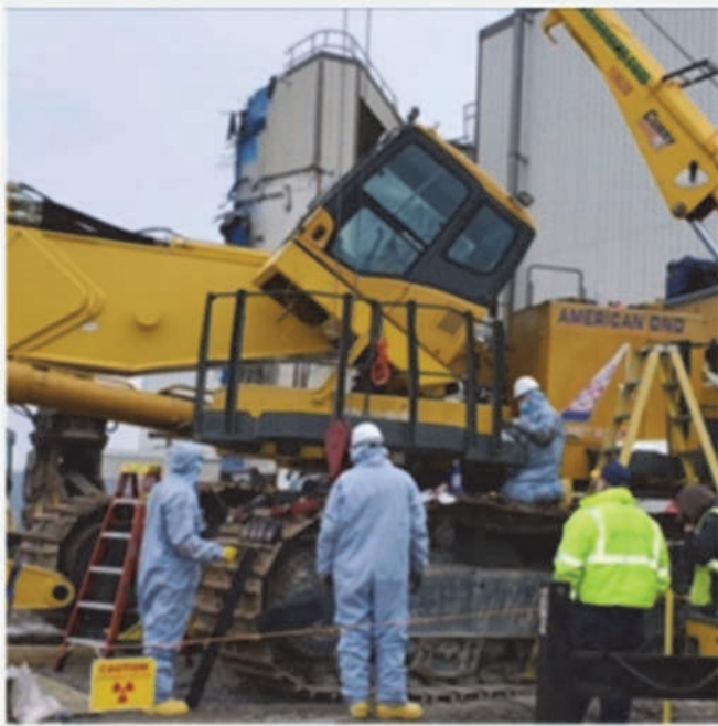
Crews install a new tilt cab in an excavator that will improve the operator's view when performing high-reach work in the demolition of the Main Plant Process Building at the West Valley Demonstration Project.
