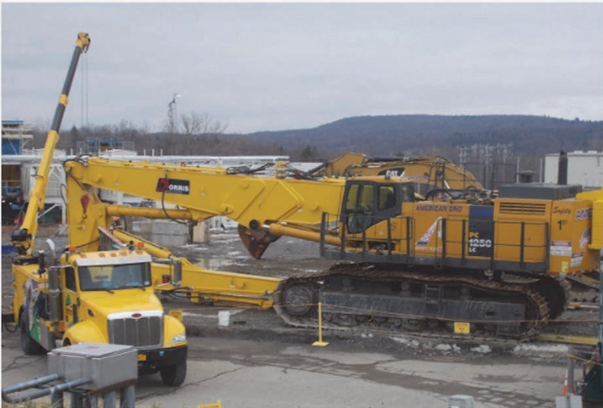
Workers at the West Valley Demonstration Project install a long-reach arm on a large excavator that will be used for the demolition of the Main Plant Process Building.
