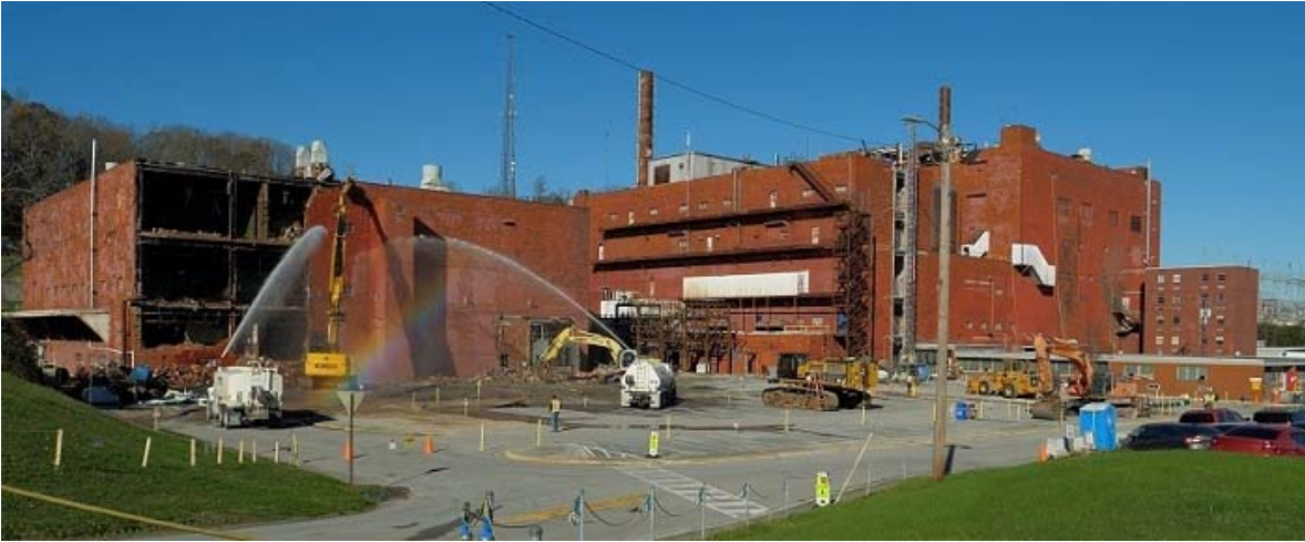
In 2021, Oak Ridge's EM program is scheduled to remove all of the remaining facilities in the former Biology Complex at the Y-12 National Security Complex. This project is eliminating buildings on DOE's list of high-risk excess contaminated facilities and clearing land for important national security missions.
