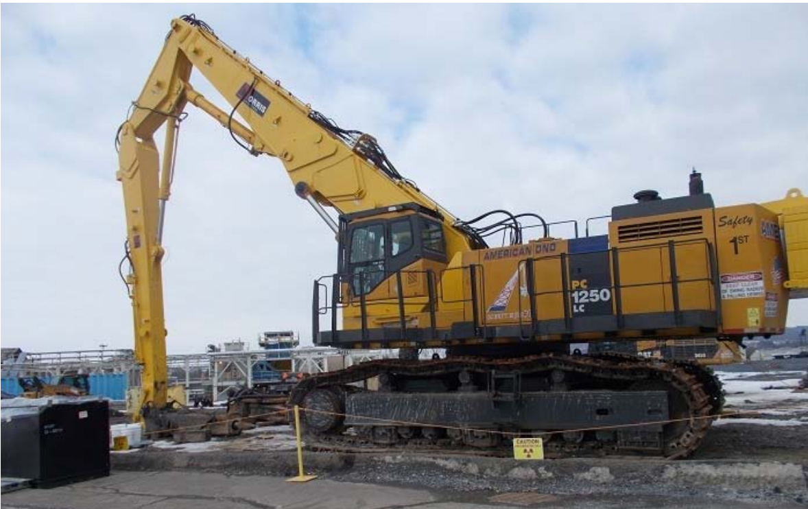
Crews at the West Valley Demonstration Project (WVDP) installed a tilt cab to an excavator, which will enable the operator to view high-reach areas by tilting the cab upward during demolition, improving safety, efficiency, and
