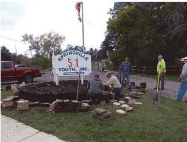
Workers from CHBWV reconstruct the bricks on the entrance sign to Springville Youth Incorporated's pool and playground area as part of their Day of Caring.
