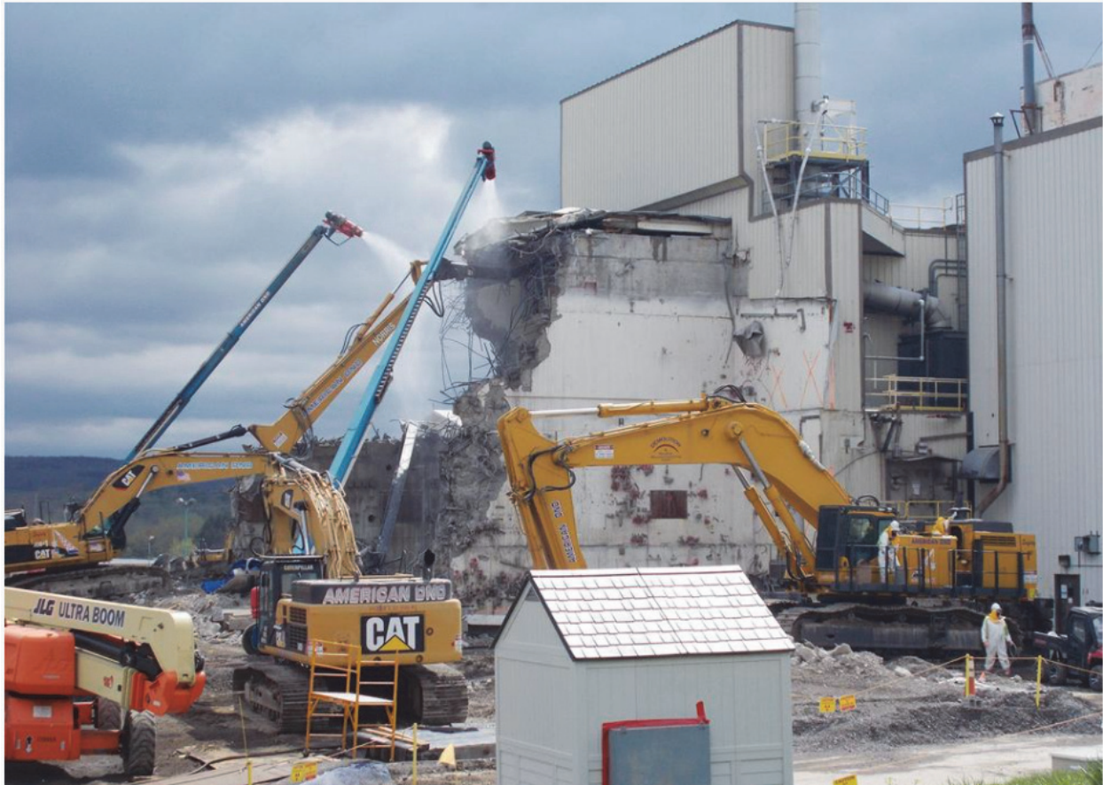
Demolition of the Vitrification Facility, a 10,700 square foot reinforced concrete structure, was completed safely in 2019 after completing waste disposition. Extensive planning and preparation were performed to prepare the facility for demolition.
