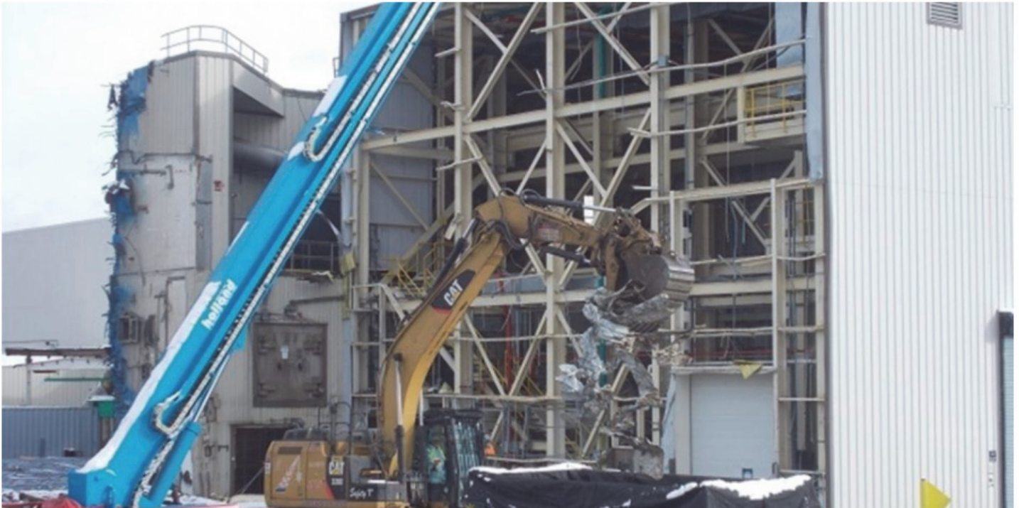
Crews take down the Load-In Facility at the West Valley Demonstration Project. The demolition is scheduled for completion early next year. (Photo: DOE)
