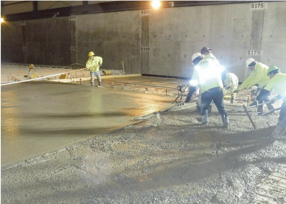
Workers at the West Valley Demonstration Project place concrete for the new floor inside the Drum Cell. The new floor will benefit waste operations during the demolition of the Main Plant Process Building, a priority for 2022.
