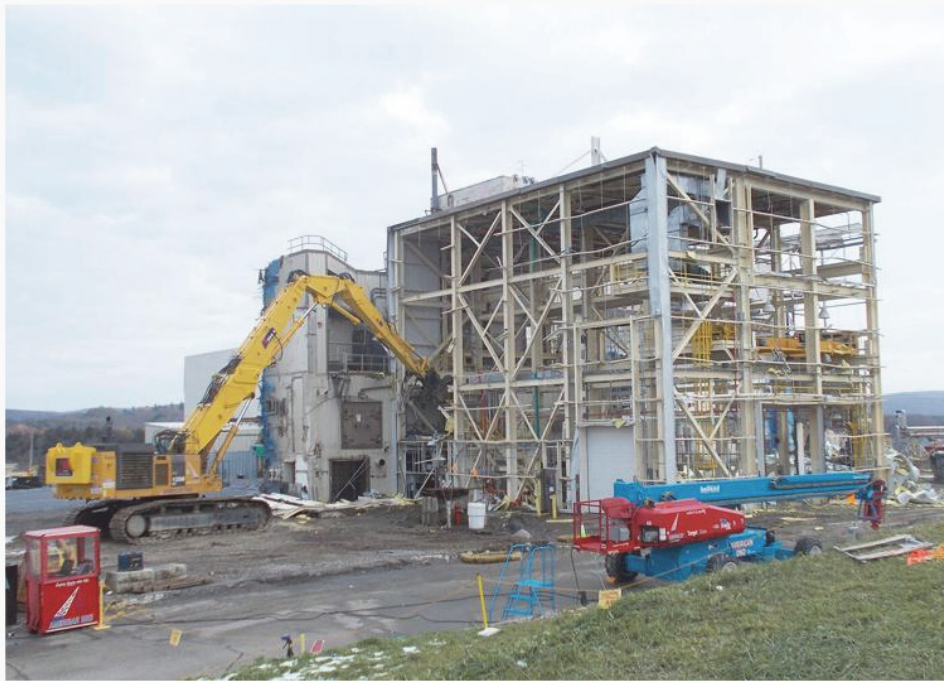
An operator uses a heavy-duty excavator to safely demolish the Load-In Facility in November 2021.
