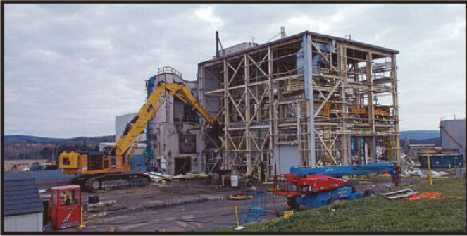
An operator uses a heavy-duty excavator to safely demolish the Load-In Facility (November 2021)
