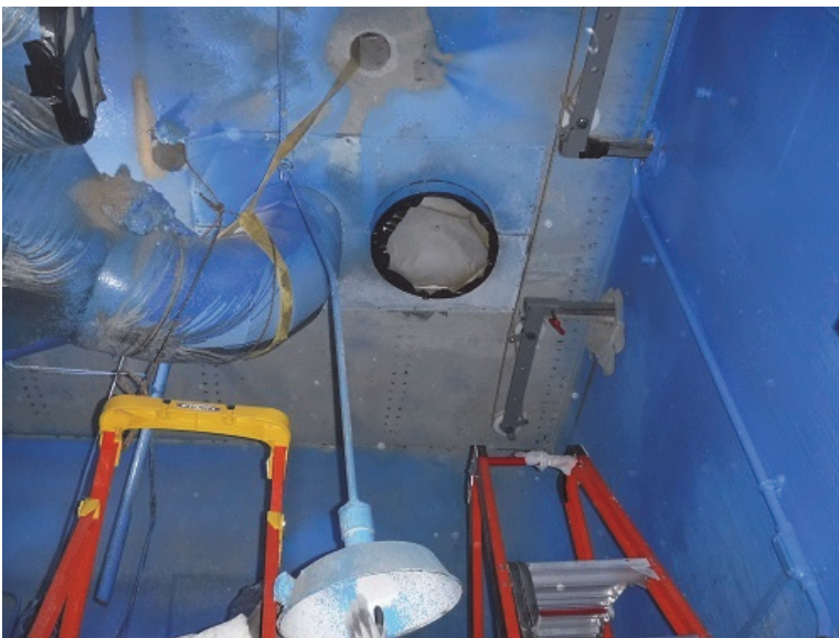
A section of a ventilation duct inside the Vent Wash Room at the Main Plant Process Building is shown before it was cut remotely with a diamond wire saw. The completed project involved 28 separate cuts to safely remove 19 sections of the duct.
