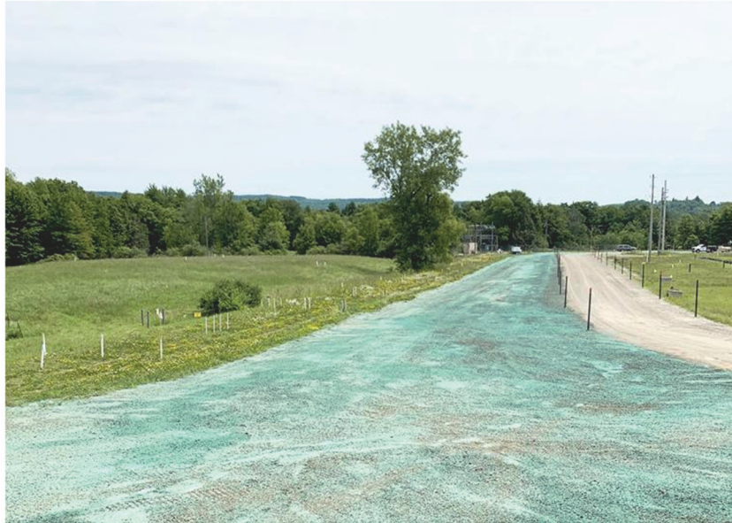
The permeable treatment wall soil and structure project area is restored with hydroseed, a technique that spreads a specialized, semiliquid grass mixture evenly over bare ground to grow grass and prevent soil erosion.
