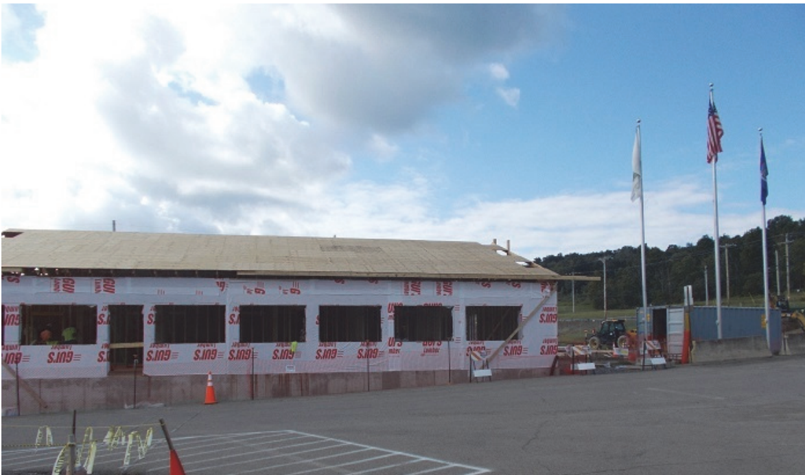
EM crews build a new security guard house at the West Valley Demonstration Project.
